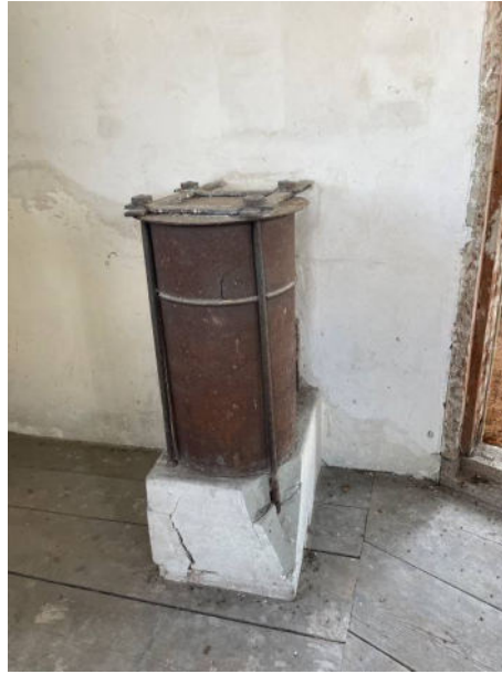
Riss in Ofensockel
